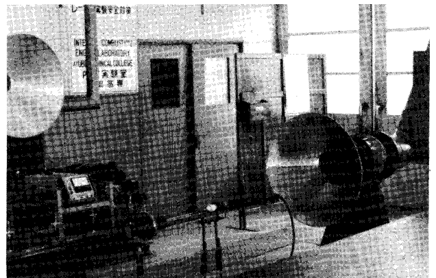
Photo. 2. An installation to draw and deliver exhaust gases.
