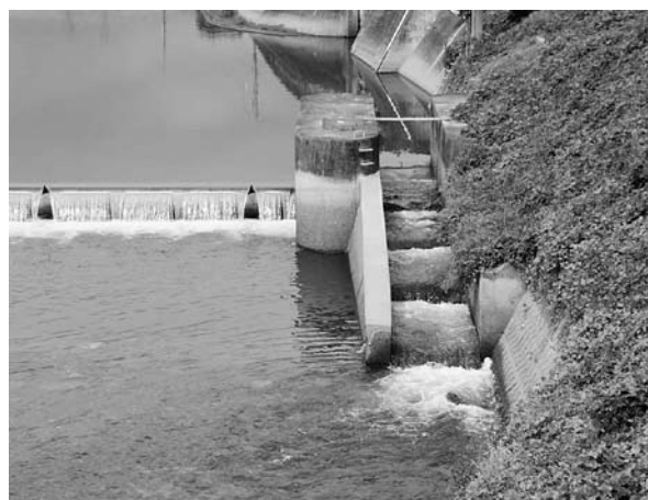
Fig. 9. Movable weirs with fishway at the Asa River in Yamaguchi Prefecture before the construction of "Mizube-no-Kowaza" fishway.
